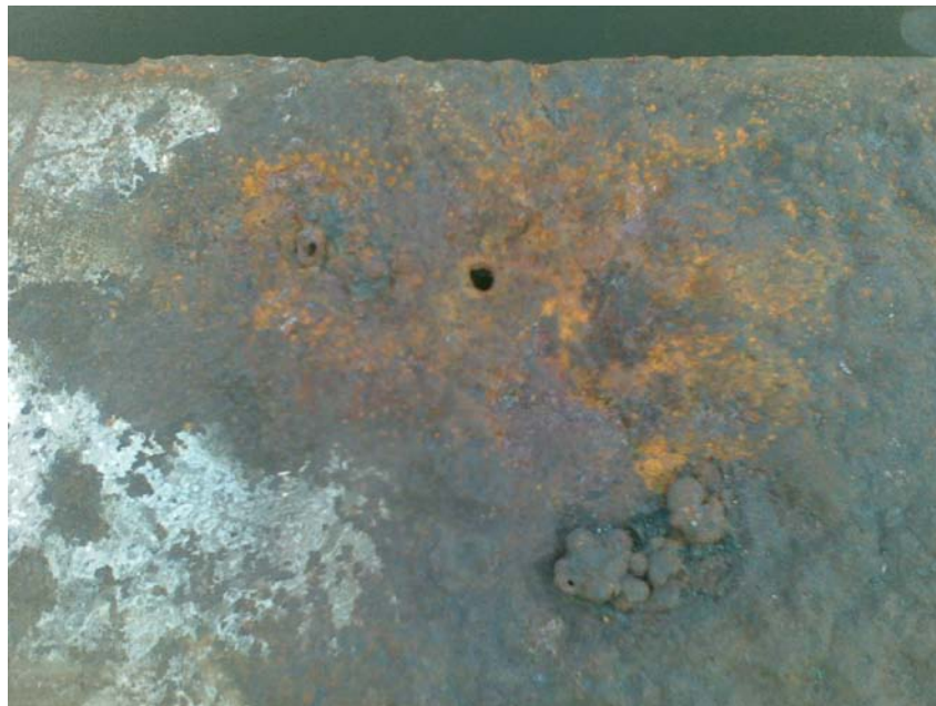
Figure 2: Soil-side corrosion on pilot project floor plate.
